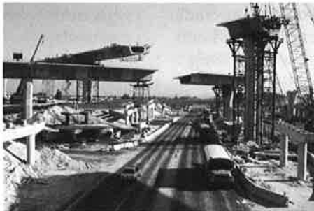
October '88 view of concrete segmental bridges being erected at I-595 and S. R. 7 interchange.
