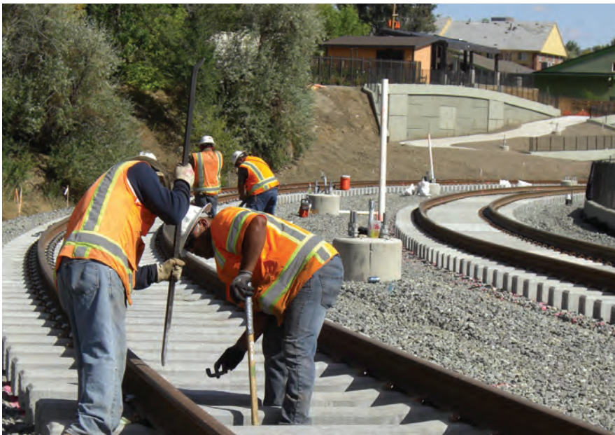
Widening the transit right of way on 13 th Avenue impacted highway crossings and homes located along the alignment.
