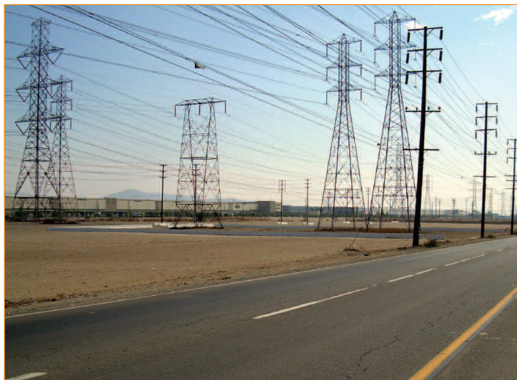
Southern California Edison has 60 acres of right of way in Unincorporated San Bernardino County.
