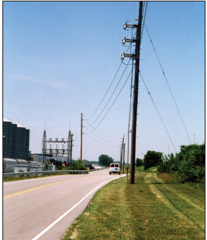
Powerline easement over a private road easement over a pipeline easement. Space is available for additional uses in the non-track area.
