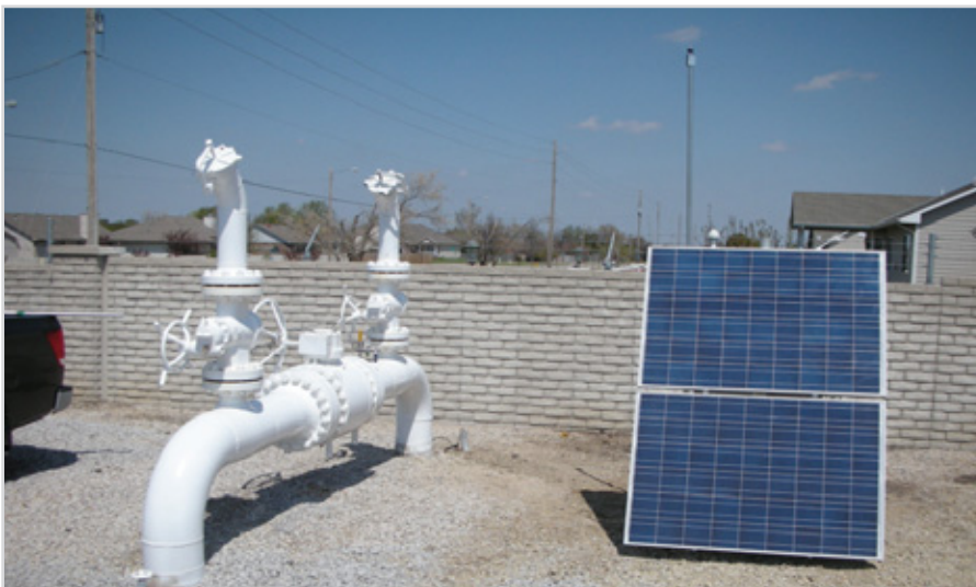
This acoustic impact detection system using hydrophone technology offers applications for natural gas, crude oil and refined products. Photo courtesy of GE Oil & Gas ThreatScan™
