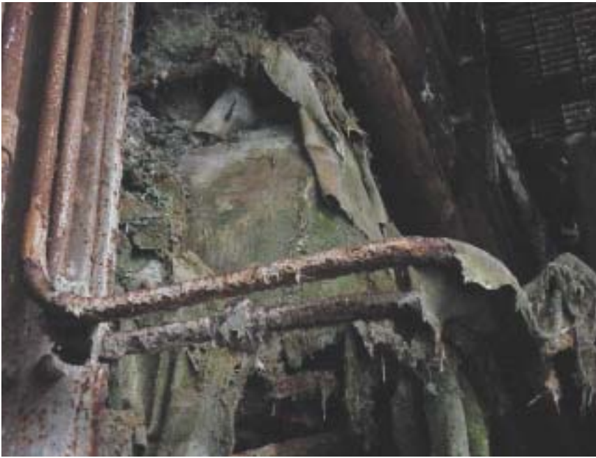
The building envelope is deteriorating. Water pours in when it rains. This has contributed to the growth of mold.
