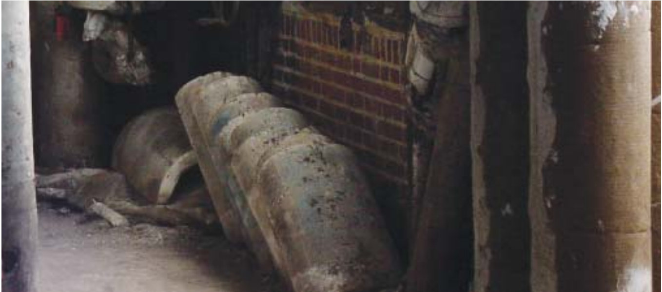
Room with a view. Semi-circles of asbestos are stacked along the floor while asbestos-covered pipes are visible in other parts of the room.
