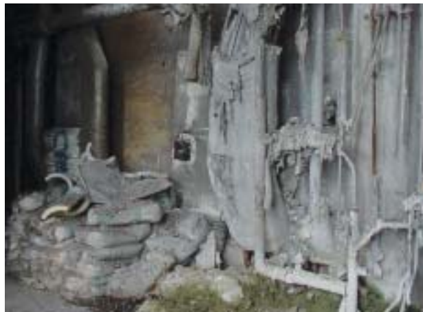
Careful not to touch the walls. Asbestos-covered material can be seen in the center of the photo. Mold is on the floor.
