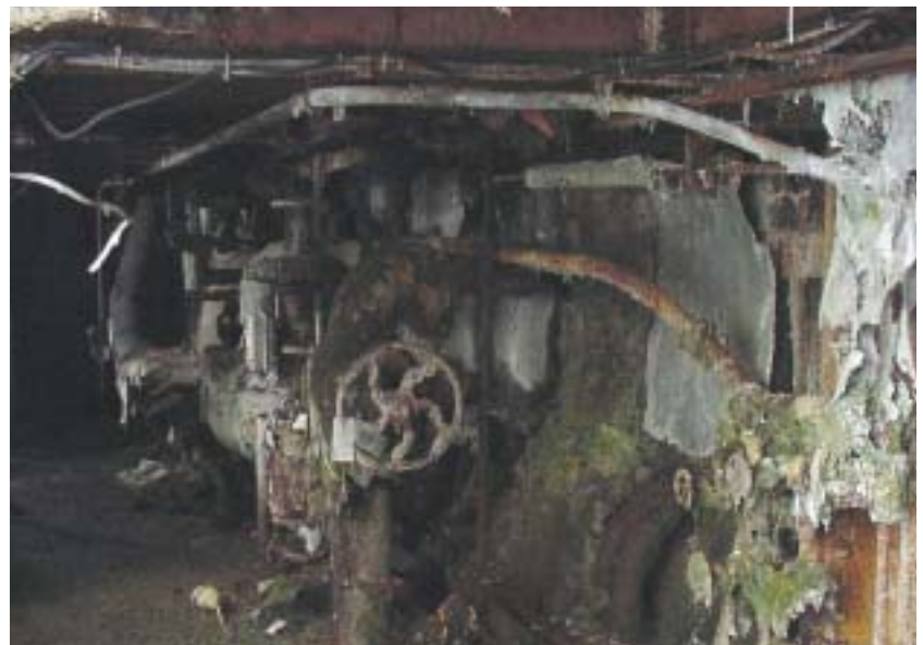
Don't track mold on the street. Mold covers parts of the asbestos remaining on the pipes while forming a goopy mix on the floor.
