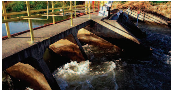
Typical canal diversion structure with remote gauging and metering system installed.
