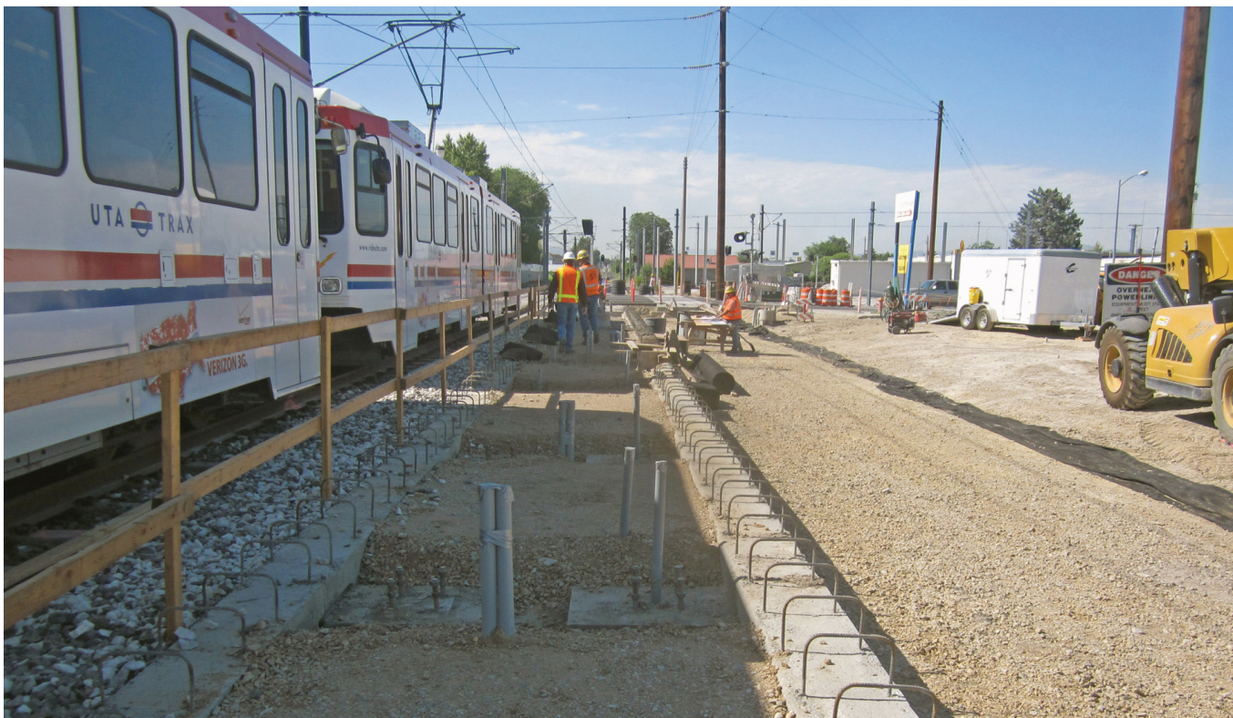
The Mid-Jordan Light Rail Transit Line was the first project to get funding and begin construction.
