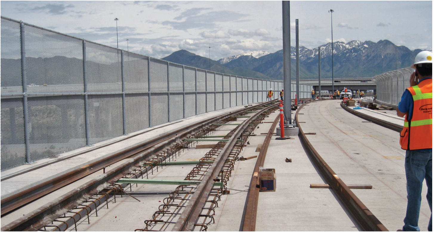
Easements proved to be far more restrictive for the West Valley Light Rail Transit Line.
