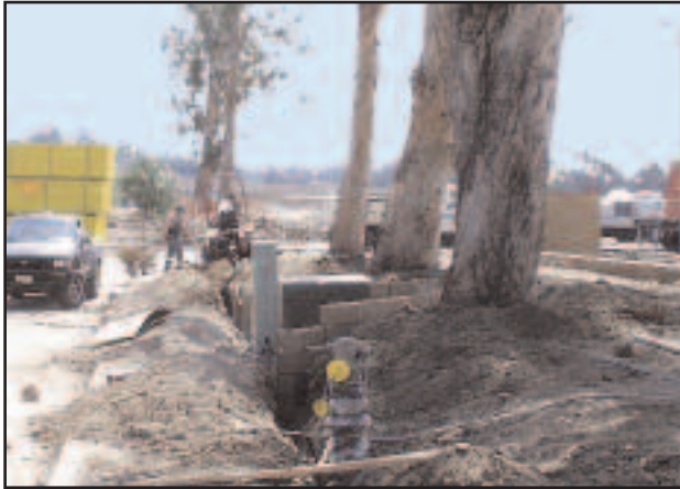
Quick and easy access to pipelines is critical.
