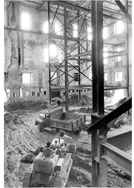
The GSA's first project was to oversee the complete gutting and renovation of the White House in 1949.
