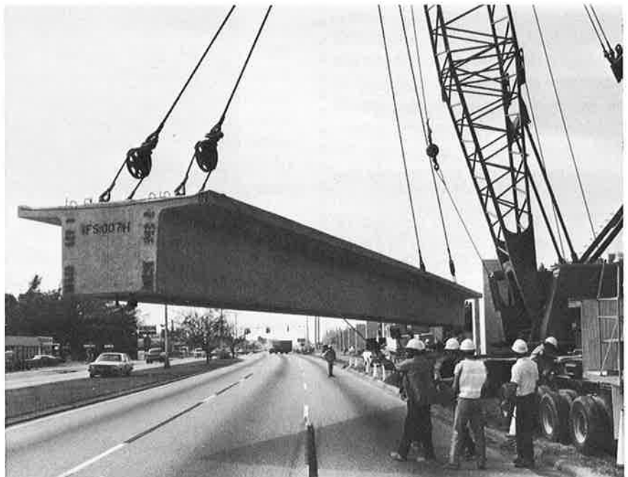
Double-Tee —One hundred tons of double-tee girder is swung into position before being lifted atop two of METRORAIL's guideway piers in South Miami.
