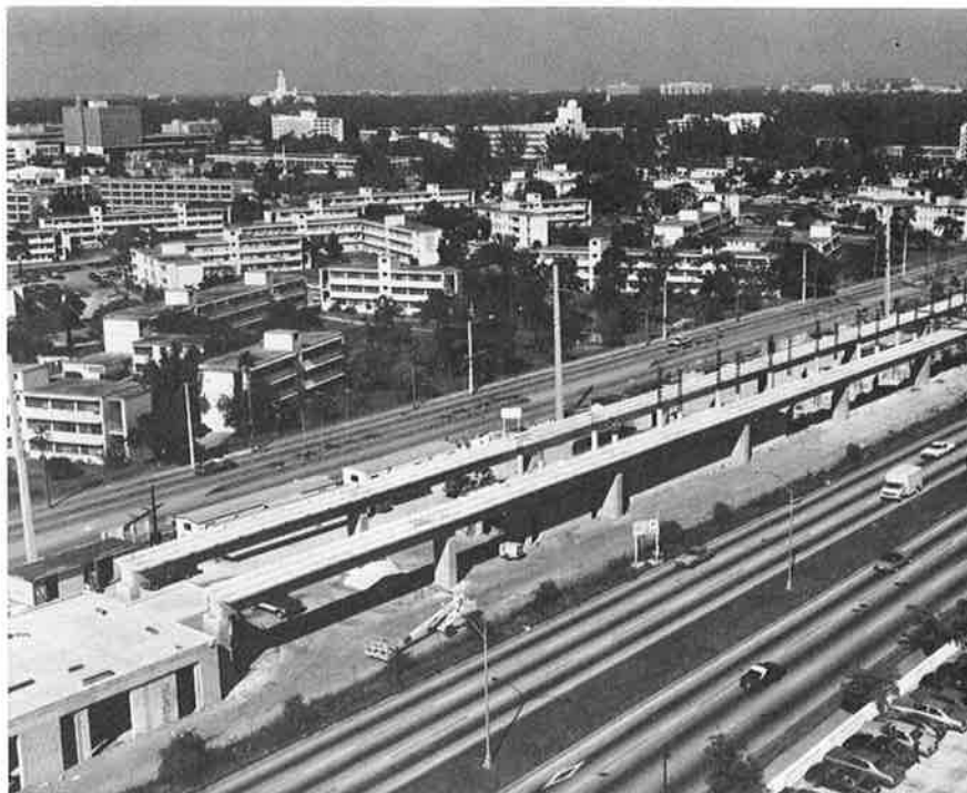
Placement —METRORAIL's 21-mile guideway begins to take shape as the placement of the first 2,330 double-tee girders is completed at the University Station site adjacent to the Coral Gables campus of the University of Miami (background).
