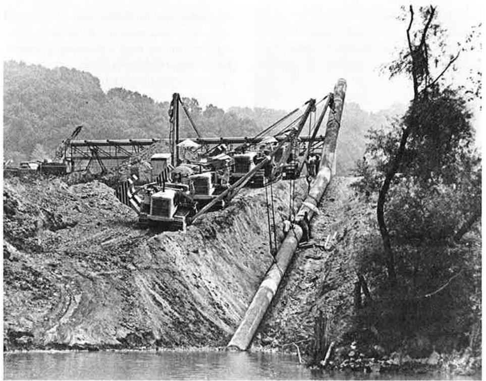
Sideboom tractors have replaced lifting poles for moving the pipeline into the ditch.
