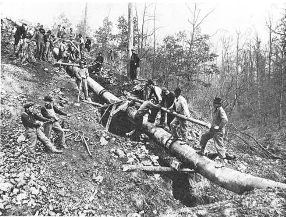
One of the first major transmission arteries of the present Columbia Gas System was this 20-inch pipeline laid in 1916 between Calendenin and Cedarville, W. Va.
