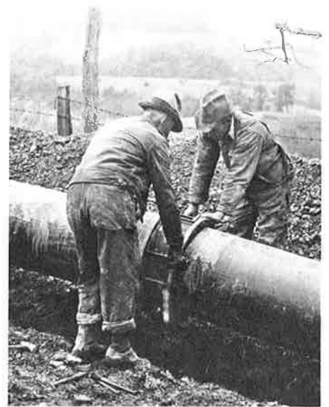
The wrench inspector working on this Columbia line in 1930 made certain all 12 bolts in each coupling were tight.
