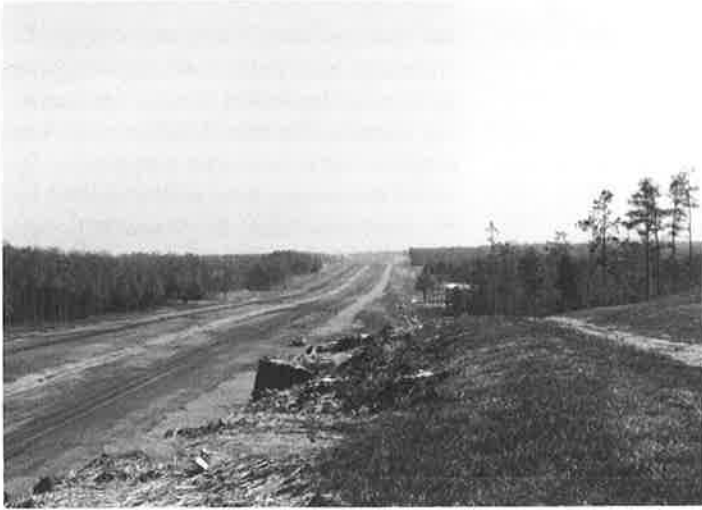
Grade and drain on new location where I-565 veered south of Alabama Highway 20 to avoid newly and heavily developed area in the town of Madison.
