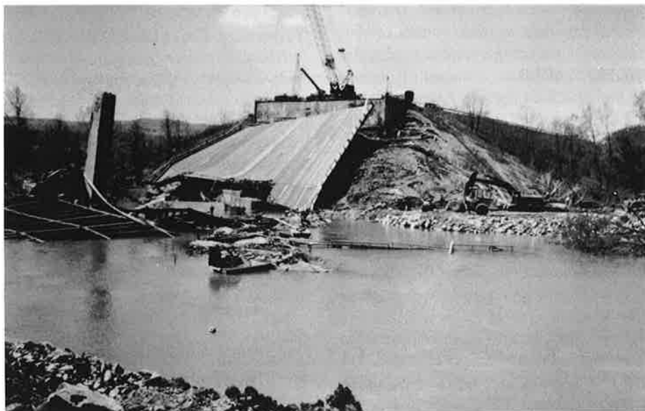
View of the collapsed New York State Thruway bridge looking west.
