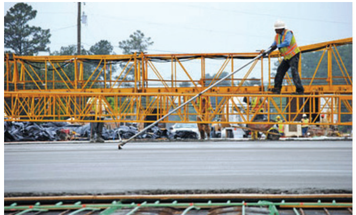
The Georgia Department of Transportation used $20.4 million in Federal-aid and state funding for the McGinnis Ferry Road extension in Gwinnett County, GA.
