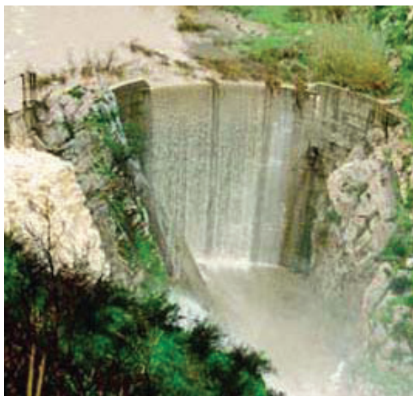
The 100-foot-high Rindge Dam was built in 1925 by May Rindge, with a 574 acre-foot reservoir to control floods and conserve the water of Malibu Creek.
