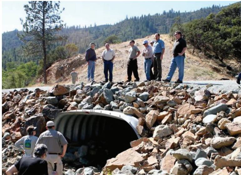
To see how projects can improve recreation access, BLM's Northwest California Resource Advisory Council visited a bottomless culvert constructed by BLM crews at Shasta Dam.
