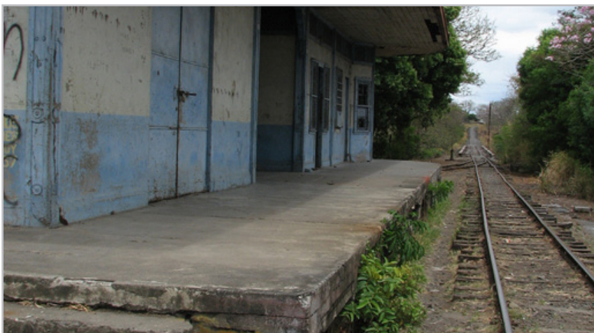
Through redevelopment programs, old abandoned train stations can be used to re-energize an inner city.
