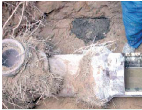
An excavated pipe penetrated by roots.
