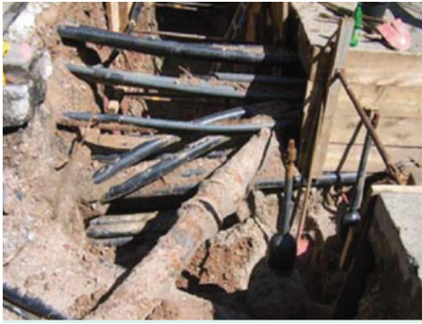
Pipelines criss-crossing the underground.
